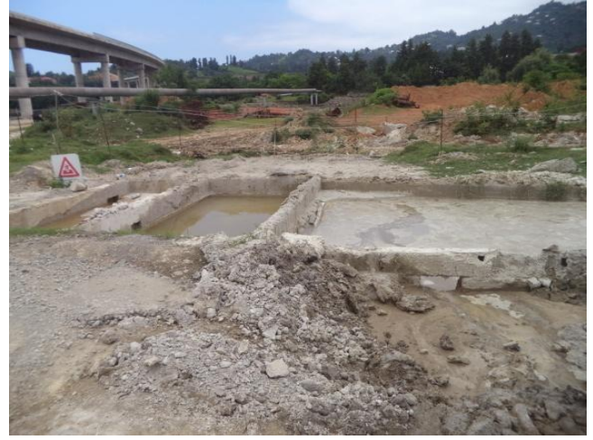
Photo 10: Basin of crushing plant is full of silt
