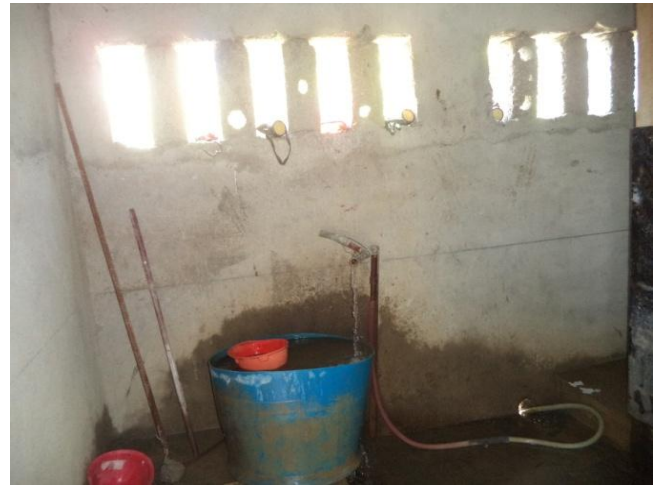
Photo 16: Taps are broken in rest rooms
