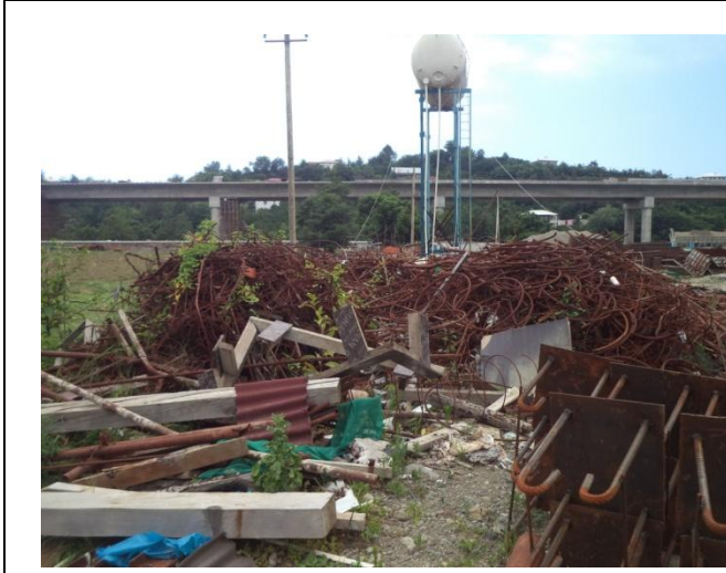
Photo 9: Scrap material accumulated on site
